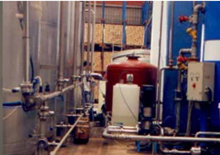
Filtration and demineralization unit
