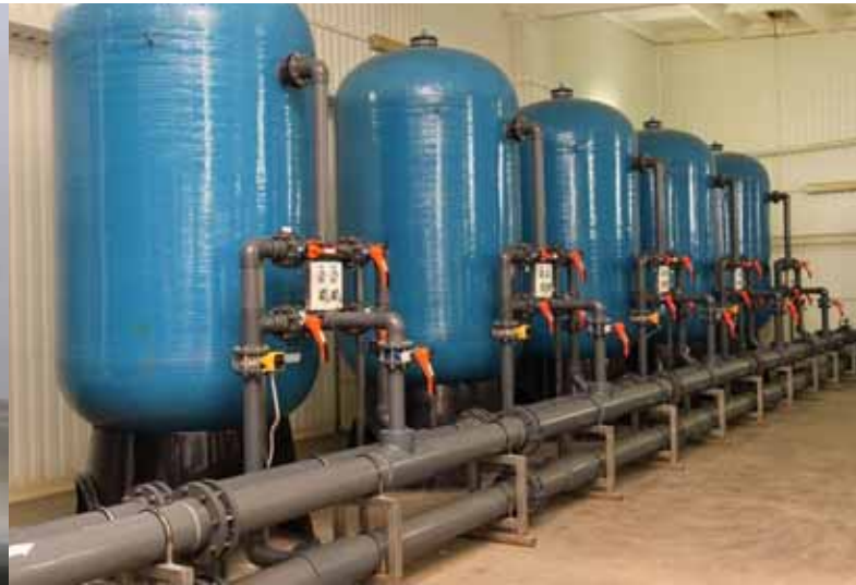
Water intermediate tank
