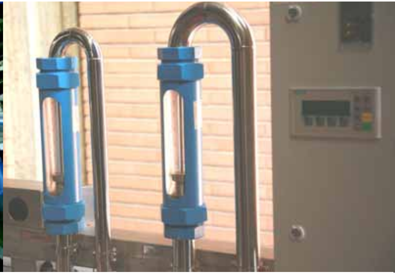
Water flow system
