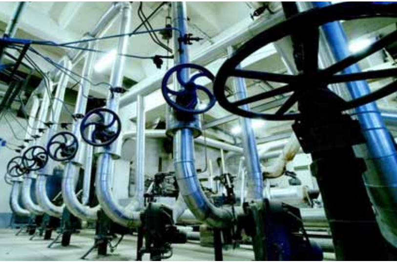
Water pumping unit
